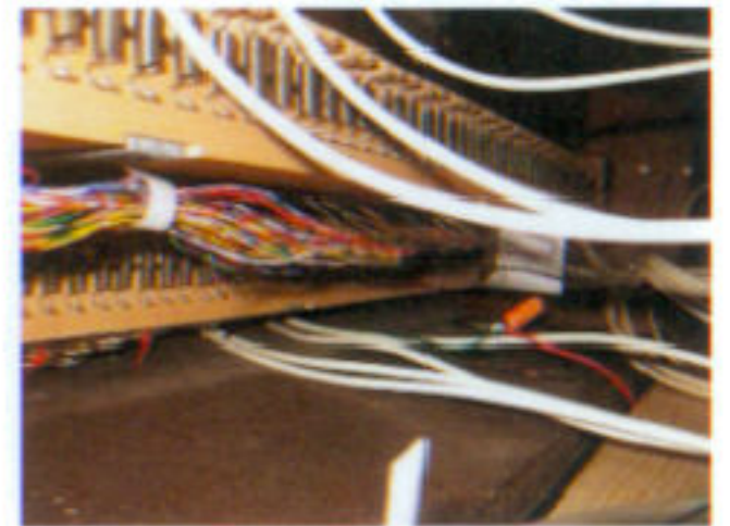
Holy Family's Organ Console Wiring
